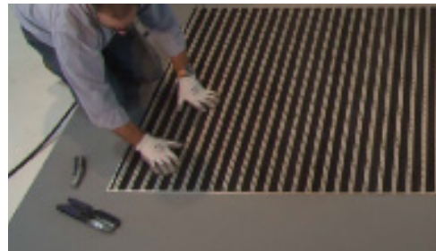
12. For beginners: we recommend using a straight edge to assist in cutting an accurate line. Once the end trim is adjusted, tuck the mat into the recess and push flat.
