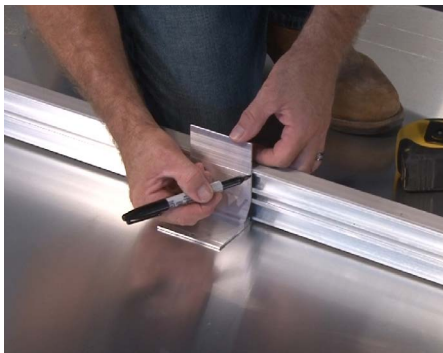
16 Place one support clip side on the floor and the other directly against the support. Use a marker to trace the support's top edge onto the clip.
