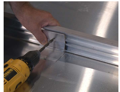
18 Use a drill to create a hole in the vertical portion of the support and the support bar behind it.
