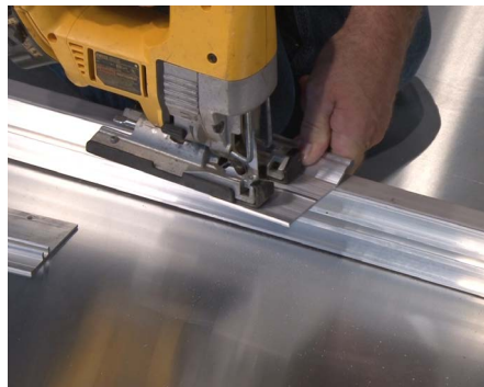
17 Use a jigsaw to cut along the transferred marker line to achieve the correct support clip height.
