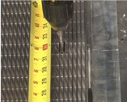
26 Using a drill or center punch tool, transfer the marked lockdown location to the I-Beam support.
