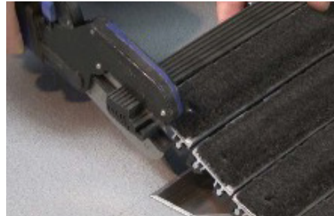
4. Cut the oversized end trim flush to the edge of the rail.
