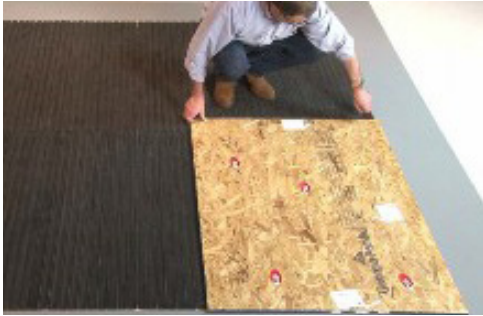
15. If construction is to continue in the building, protect the unit with plywood sheathing.
