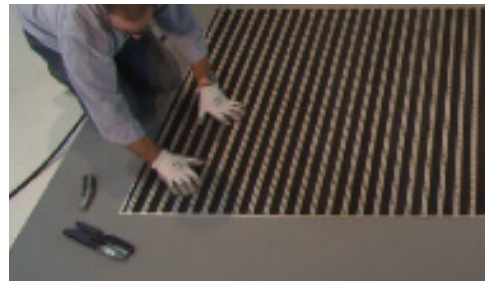
6. For beginners: we recommend using a straight edge to assist in cutting an accurate line. Once the end trim is adjusted, tuck the mat into the recess and push flat.
